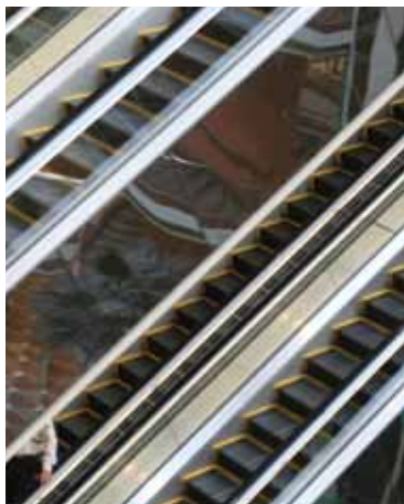
Lifts Passenger transport
